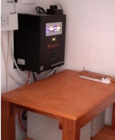
New solar system
